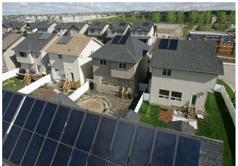
Solar panels on the roof of low-rise development.
